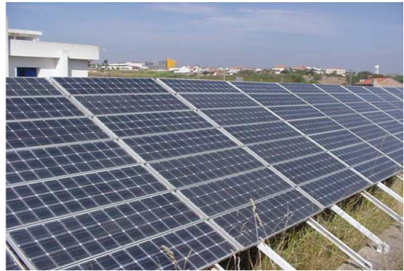
Figure 2.4: Panneau photovoltaïque fixe
