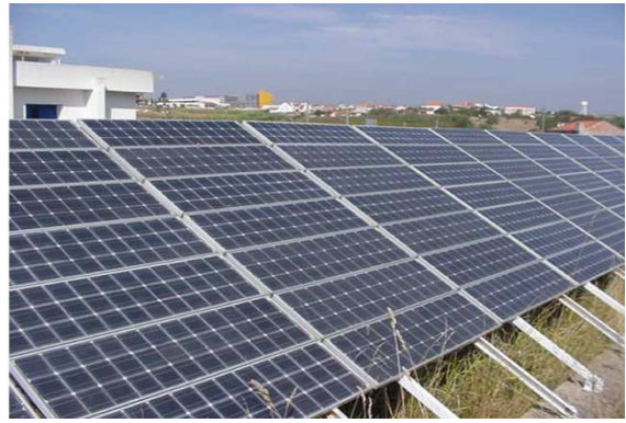
Figure 2.4: Panneau photovoltaïque fixe
