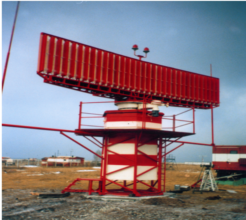
Figure 2.6 Antenne radar secondaire
